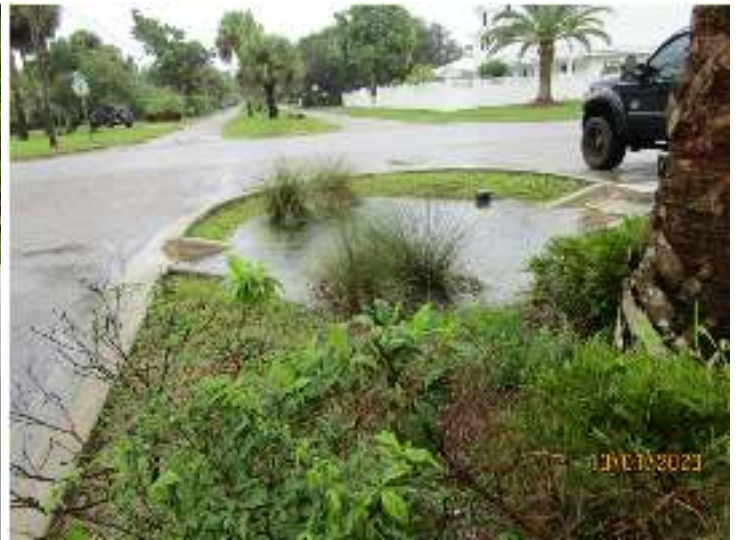
Sunset at Pine – After we completely cleared and cleaned the entire swale median water collects and stays in the swales.
