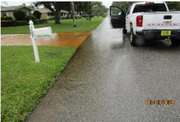
Poinsettia – East End – No functioning underground pipe. The water floods the yards along the street.
