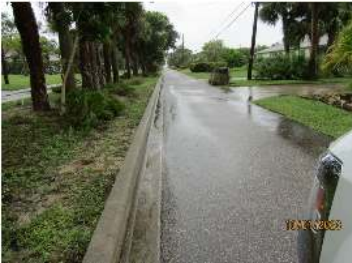
Sunset to the West – Prior to our cutting the curbs this area held water for a long period.
