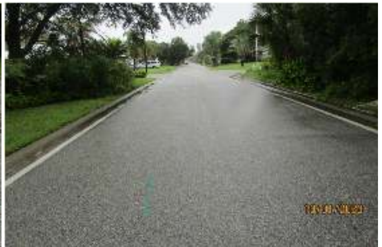
Pine and Second – Note that less water is flowing on the west side of the road. That is attributed to our having built a small swale at First and Pine.
