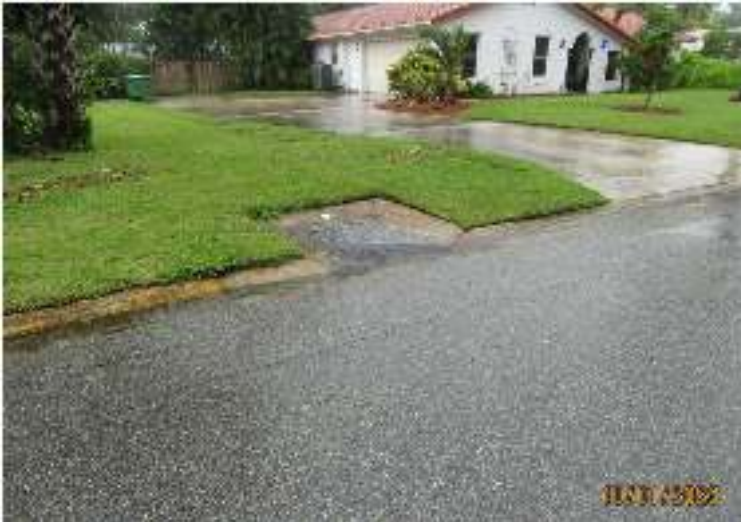
Drain Inlet on S. Palm – A line from Flamingo crosses through the properties here and feeds that water into this inlet. That renders this inlet useless for water traveling south on the west side of S. Palm causing yard flooding to a nearby residence. It has nearly entered that garage in the past
